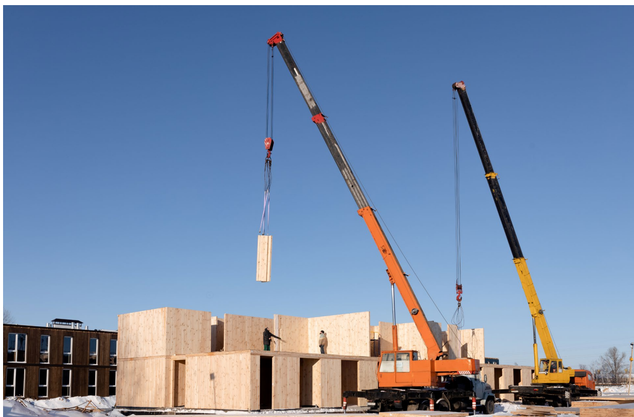
Construction of homes with cross laminated timber in Chernihiv for residents who lost their homes due to Russian aggression. 2023. Source: CLT Rezult ( https://clt-rezult.com/ )
