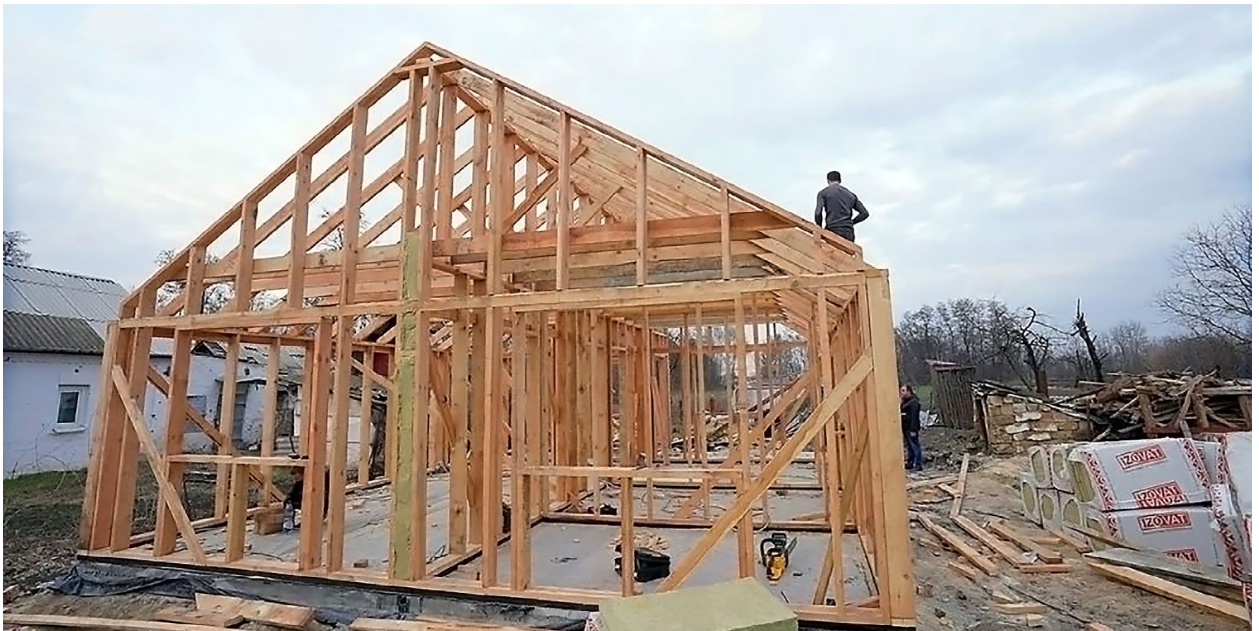
Restoration of destroyed homes in the Novobasanska Consolidated Community, Chernihiv Oblast, 2023. Source: Suspilne Chernihiv
