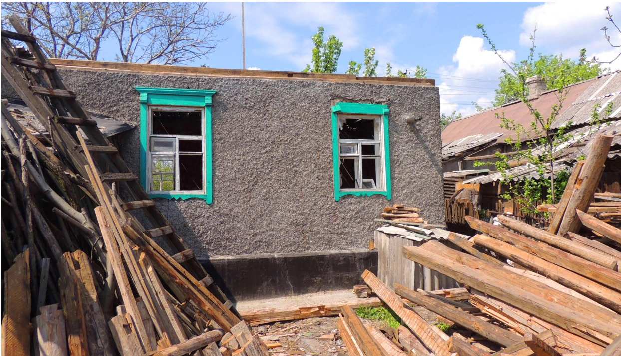
Repairs to traditional village homes damaged during Russia’s first invasion of Ukraine, 2015. Nizhne, Luhansk Oblast. Source: Brian Milakovsky
