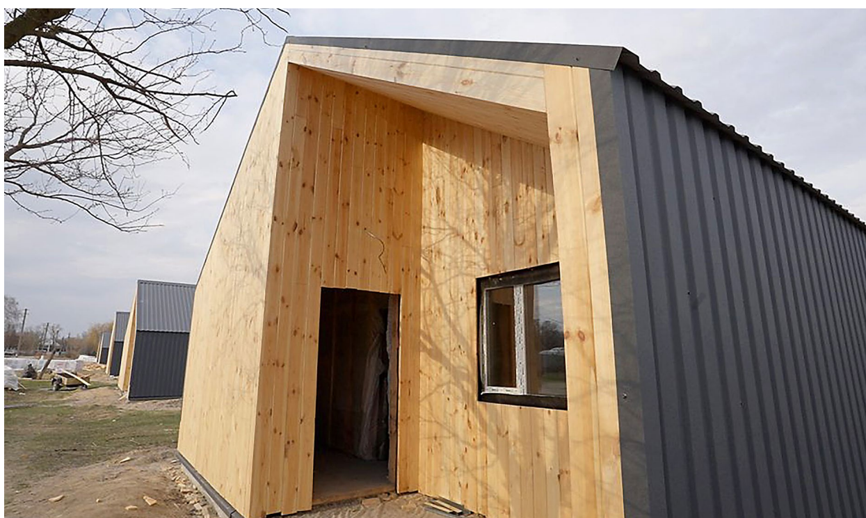
Construction of wooden homes in Stariy Bykiv village (Chernihiv Oblast) for residents who lost their homes as a result of Russian aggression. 2023. Source: Suspilne Chernihiv
