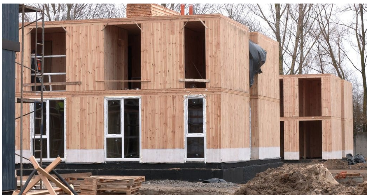
Construction of wooden homes in Chernihiv for residents who lost their homes due to Russian aggression, 2023.
